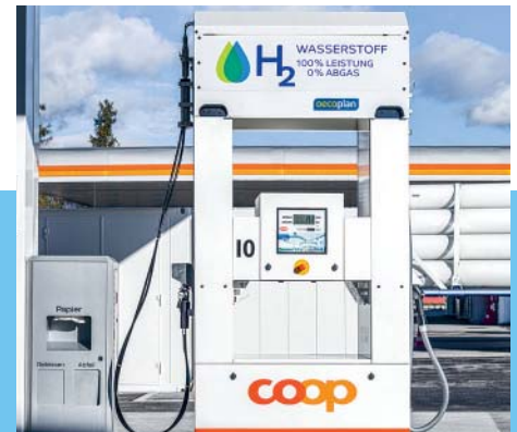
Coop hydrogen dispenser
